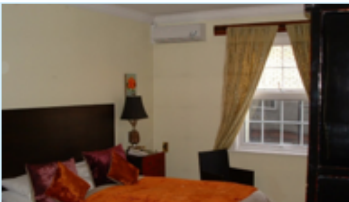
Air to Air Heat Pump Wall Unit
